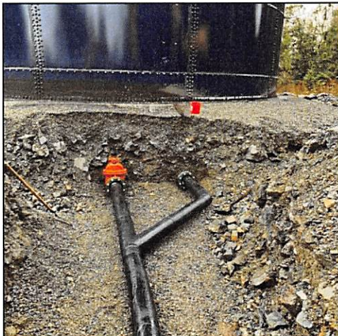
Reservoir Drain / Overflow Piping
